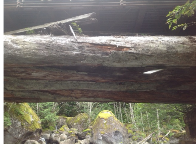
old log stringers underneath
